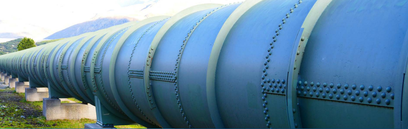
Water pipeline. Photo: LoggaWiggler
